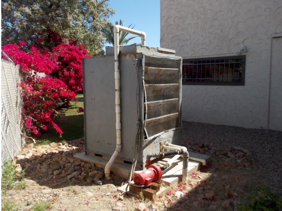
Deferred maintenance – water tower unit.
